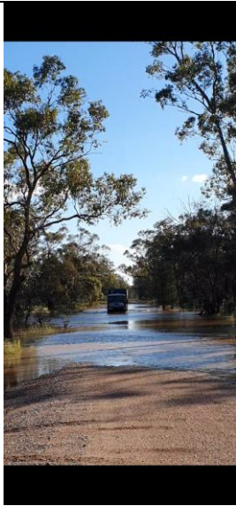
Plate A6.7 – Floodwater inundating the Tubby Lees Road causeway crossing of Gunningbland Creek.
