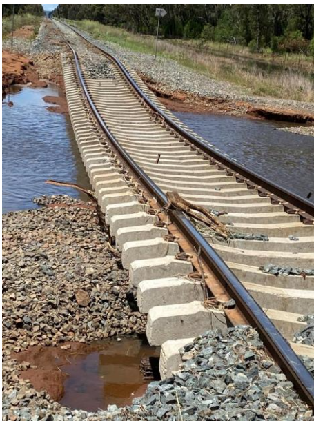
Plate A7.20 – Collapsed section of railway immediately to the east of Overland Road.
